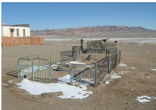
Photo 1. Outdoor protected well in rural area
